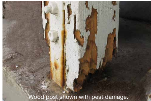
Wood post shown with pest damage.
